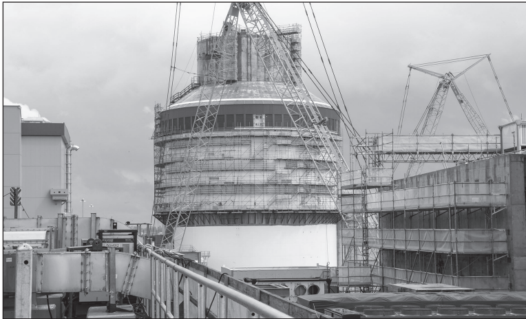
Experts for the Georgia Public Service Commission are predicting that Vogtle construction will require two years and $2 billion more than Georgia Power says. Georgia Power claims that the reactor will be on-line later this year while also admitting that they are having to re-do faulty electrical wiring. Progress on the Nuclear Regulatory Commission safety review is extremely slow-going with more than half of the nearly 400 items that must be checked off remaining unfinished. March 2021 Vogtle 3 containment, photo courtesy Georgia Power
